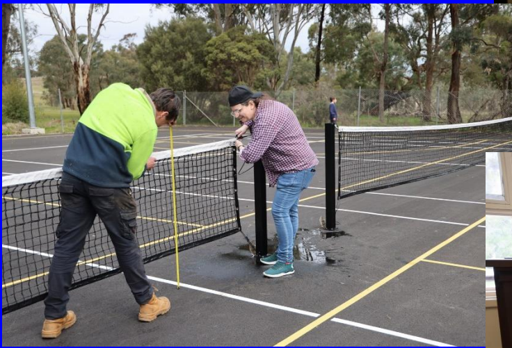
Above : There were tennis court nets to erect on the newly surfaced tennis and basketball courts. Here Bronwyn Fanning from Rotary Altona City helps Benji.
